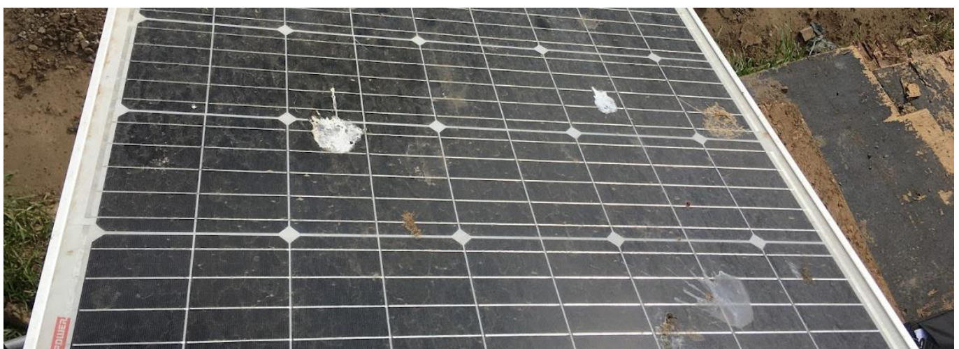
Even mild fouling of a solar panel can be enough to completely impair its function. Image source: UTS.
