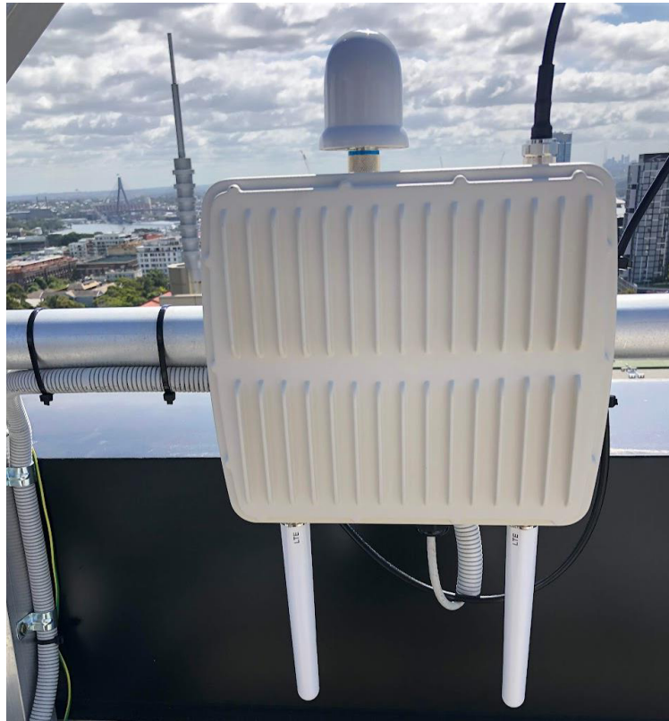
A communications gateway can fail for a wide range of reasons, resulting in partial or complete loss of network communications. Image source: UTS.
