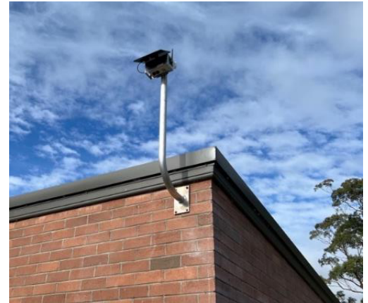
A J-pole extension installed in Sutherland Shire (NSW) for the purpose of mounting a Clarity air quality sensing device.
