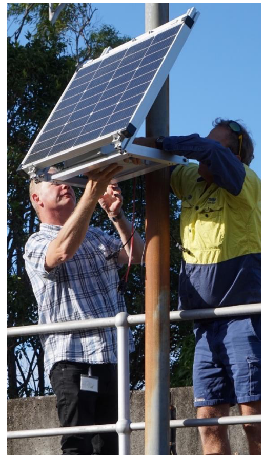
Installation of an air quality sensing device and solar panel in Tweed Heads, NSW. Image source: Tweed Shire Council
